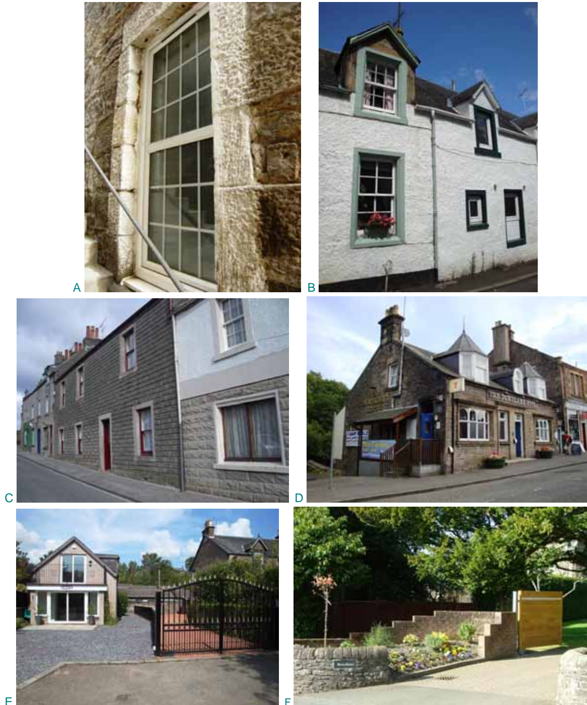
Fig 25A: uPVC replacement window inserted into traditional stone opening, the materials are unsympathetic for the historic building and the mock astragals do not follow original patterns or detailing; B: compare the effect on the appearance of the building of original windows (left) with inappropriate replacements (right); note also the modern cement based rendered and painted walls; C: mock stone facing to buildings in High Street is visually detrimental and could cause problems for the building fabric; D: small changes such as the side porch on the Dunblane Hotel, can erode the good quality of the rest of the building; the satellite dish is also poorly sited; E: boundary enclosures and road, pavement and drive finishes are important.
